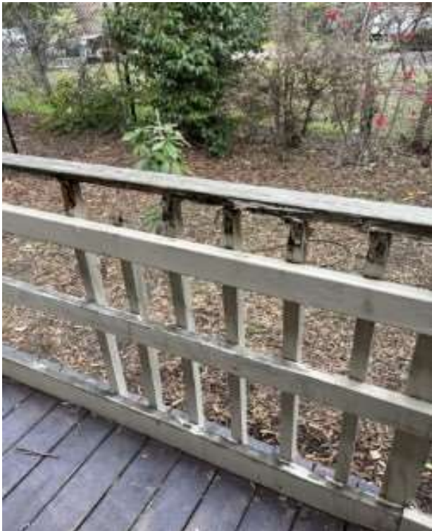
Rotted handrail outside Bldg. 2
