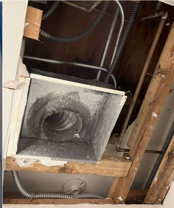
View of the bathroom ceiling in Bldg. 1
