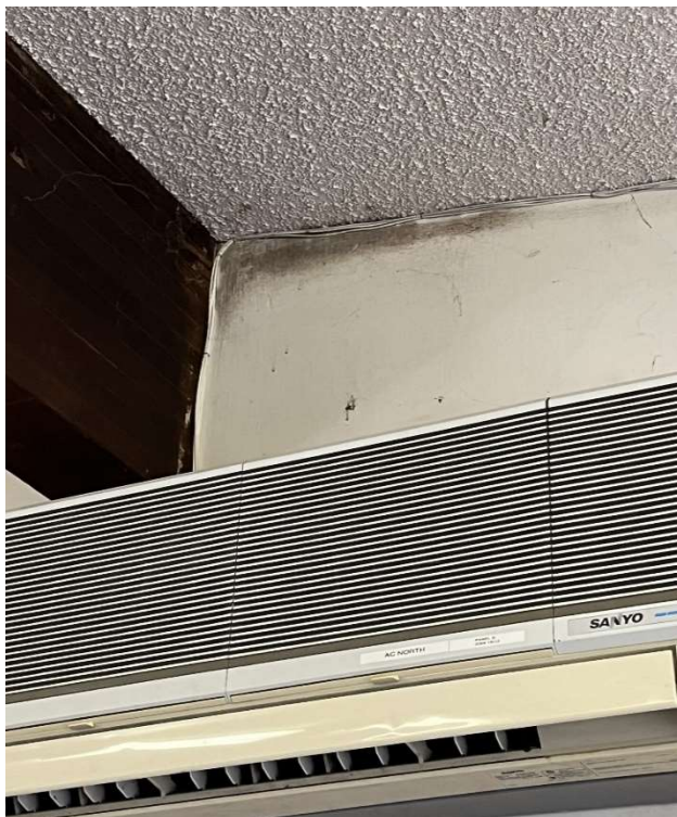
Evidence of water intrusion and possible mold in Bldg.2
