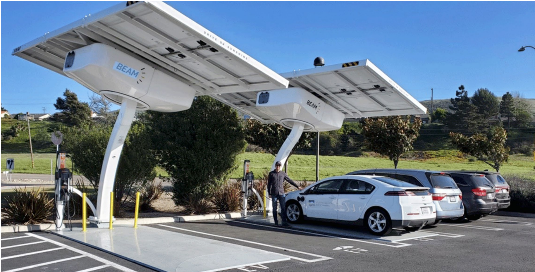
BEAM EV Arc mobile charging stations are powered by solar panels and battery systems in Lompoc
