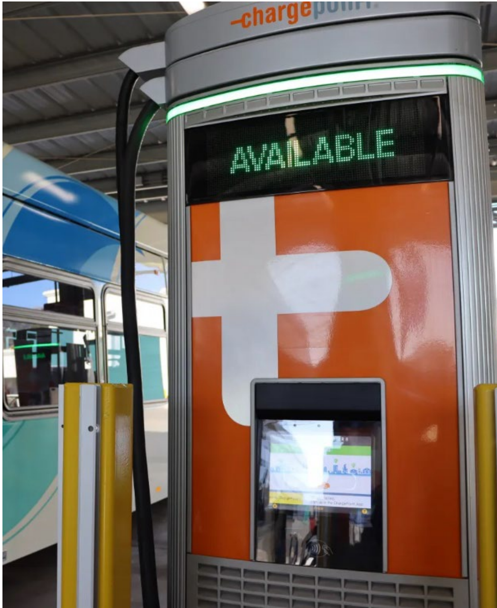
Fast charging station at Santa Barbara Metropolitan Transit District bus depot
